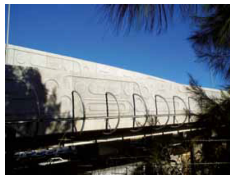
Figure 3: Glebe Island off-ramp, Australia – GRC reflective barriers.
