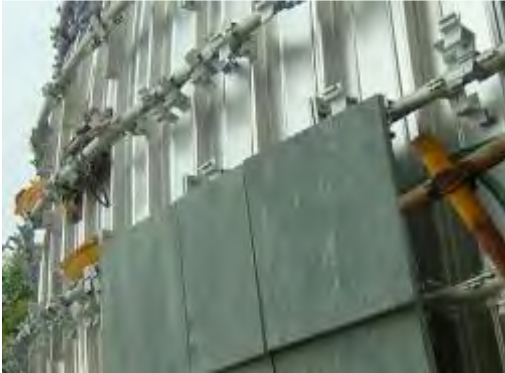
Figure 4: Facade under construction at the China Academy of Fine Arts showing a stone architectural finish clipped to a substrate. Image courtesy Tony Mills.
