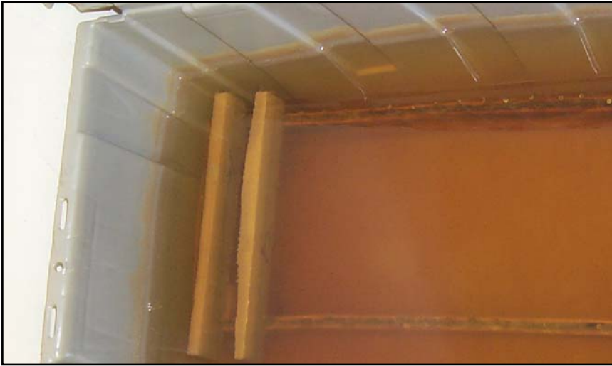
Figure 3 – Test Coupons Placed in racks inside the Hot Water Tank
