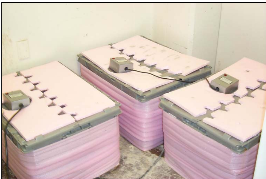
Figure 2 – Hot Water Tanks with Water Temperature Controls
